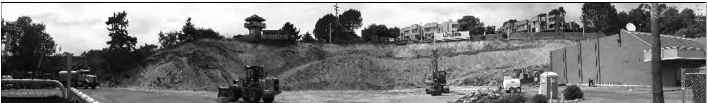
Flower Hill Changes: stop work order posted - theater closed - hillside devastated - old growth trees killed www.stopflowerhill.com
